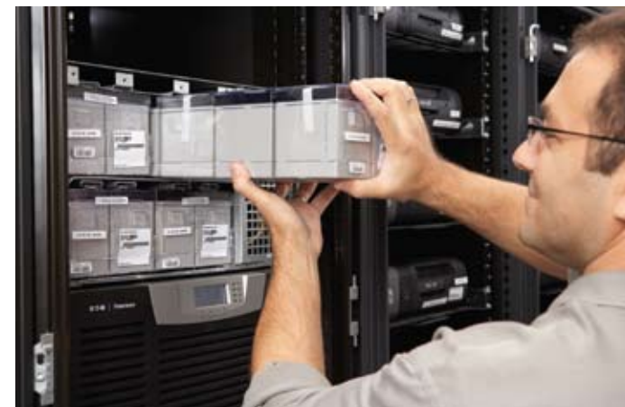
IT staff can easily replace battery modules.
