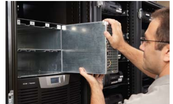
IT staff can easily install electronics modules.
